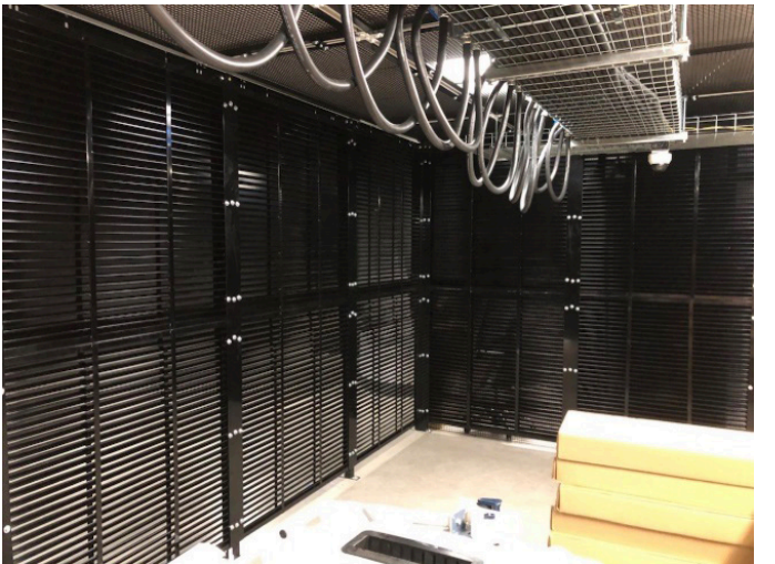
INSIDE VIEW OF LOUVER SYSTEM
