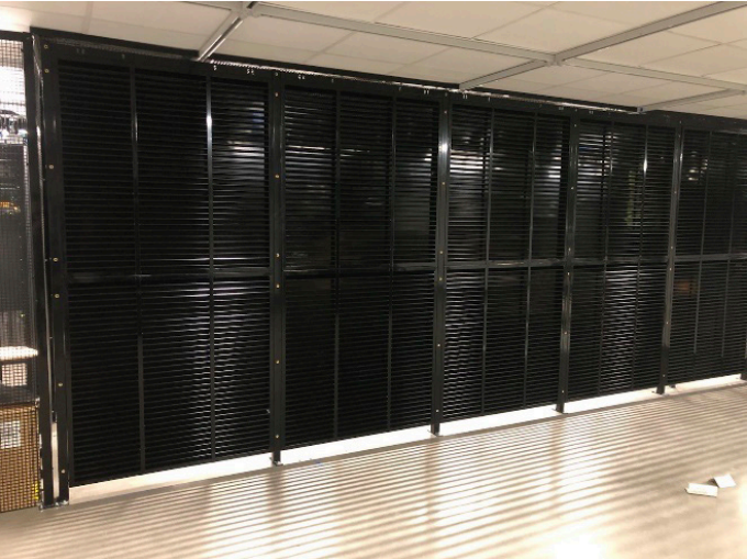
OUTSIDE VIEW OF LOUVER SYSTEM
