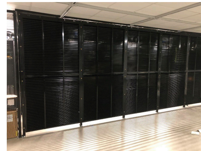
OUTSIDE VIEW OF LOUVER SYSTEM
