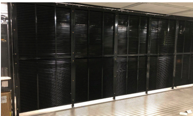
Outside View of Louver System
